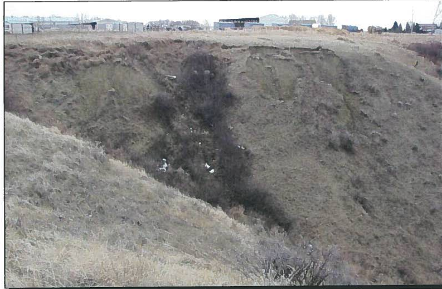
Photo 4 Skin Failures on North Perimeter Slopes (Looking South)
