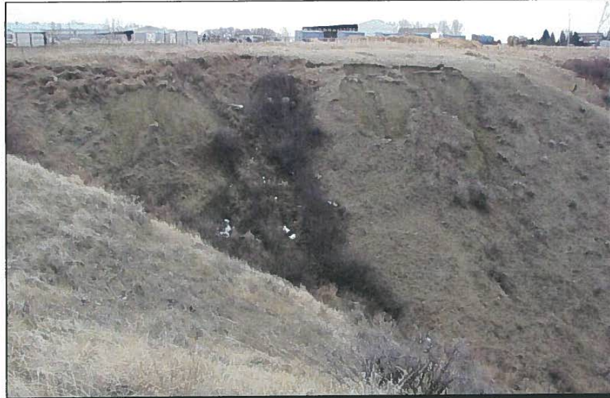
Photo 4 Skin Failures on North Perimeter Slopes (Looking South)
