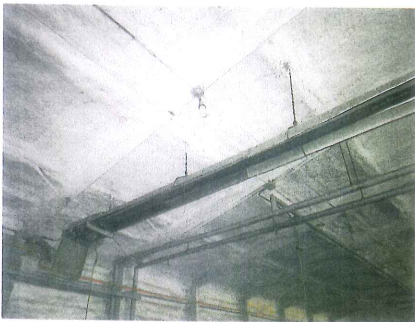
Photograph 2: - View of the spray on insulation and radiant heat in barn area.
