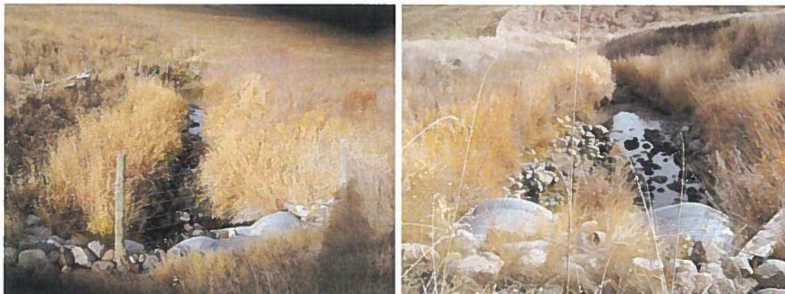
Figure 1 – Upstream (left) and Downstream (right) Ends of Highway 25/Piyami Coulee Culverts (Photo by MGCL, 23 October 2007)
