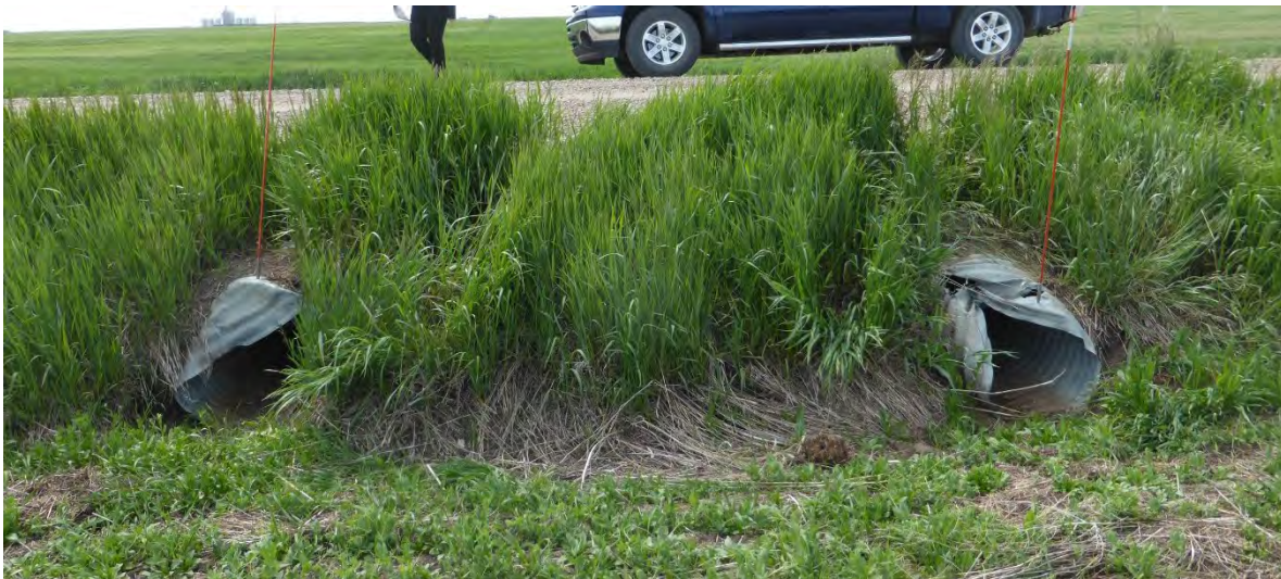
Collapsed Culverts- Upstream Tiffin Drain
