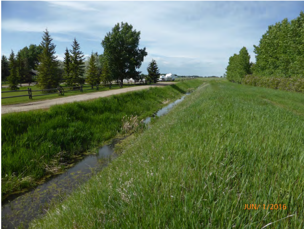
Tiffin Drain - Good Condition, North of Highway 508
